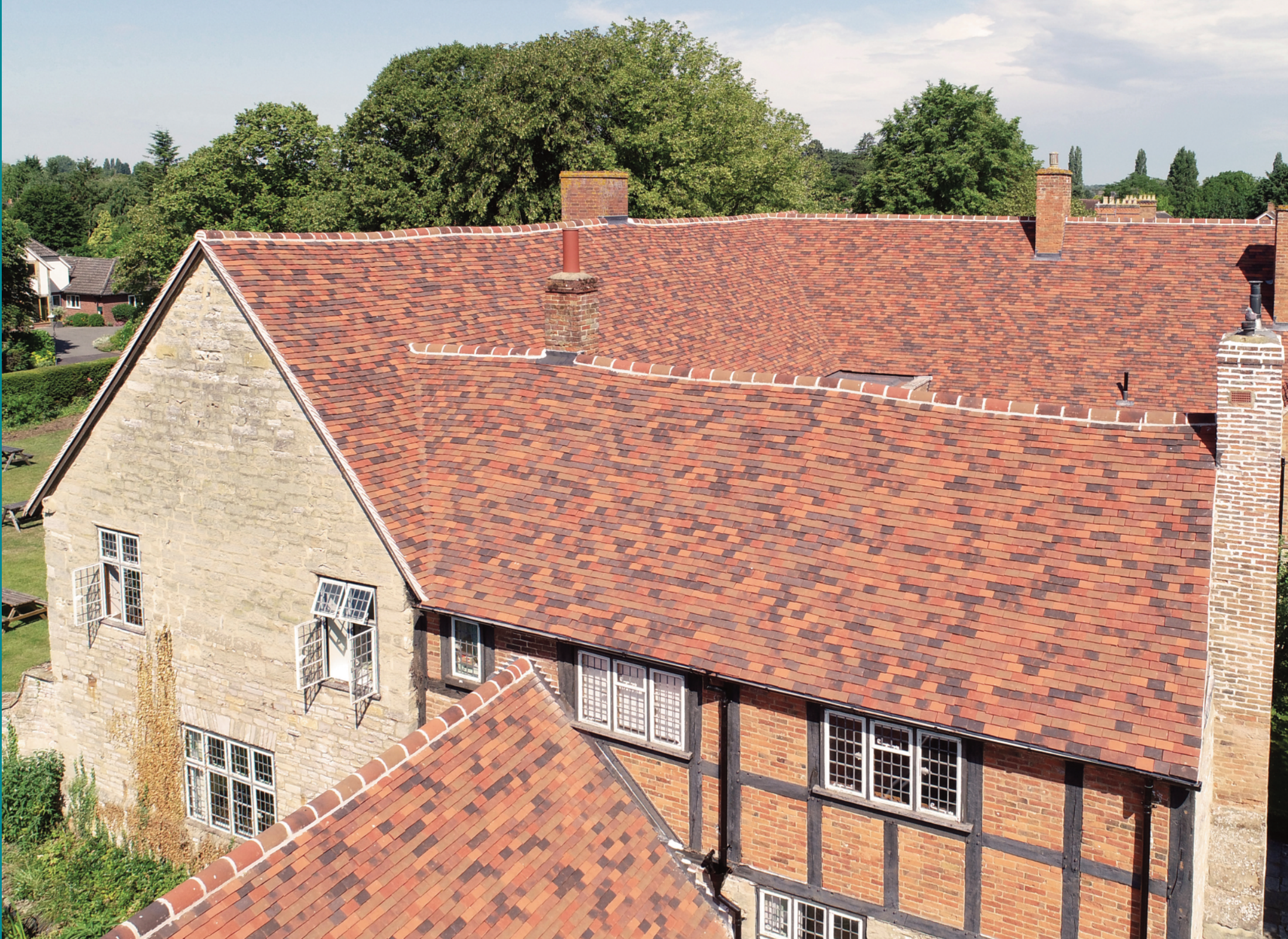
Grade II listed building Roof: Seven Colour mix - Dark, Medium & Red Antique, Sussex Red & Brown, Jubilee, Weathered Earth
